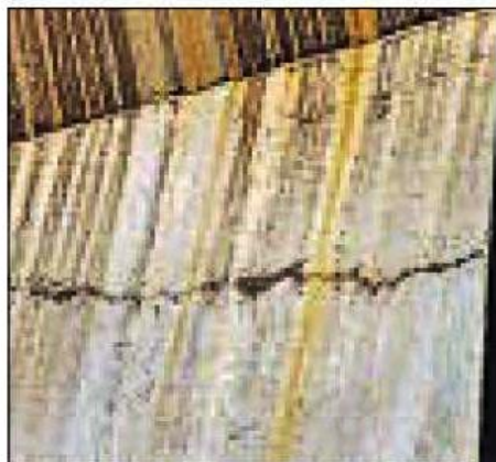
■ Cracks in a pillar near the Ramakrishna Ashram Marg Metro station. SUNIL SAXENA/HT
